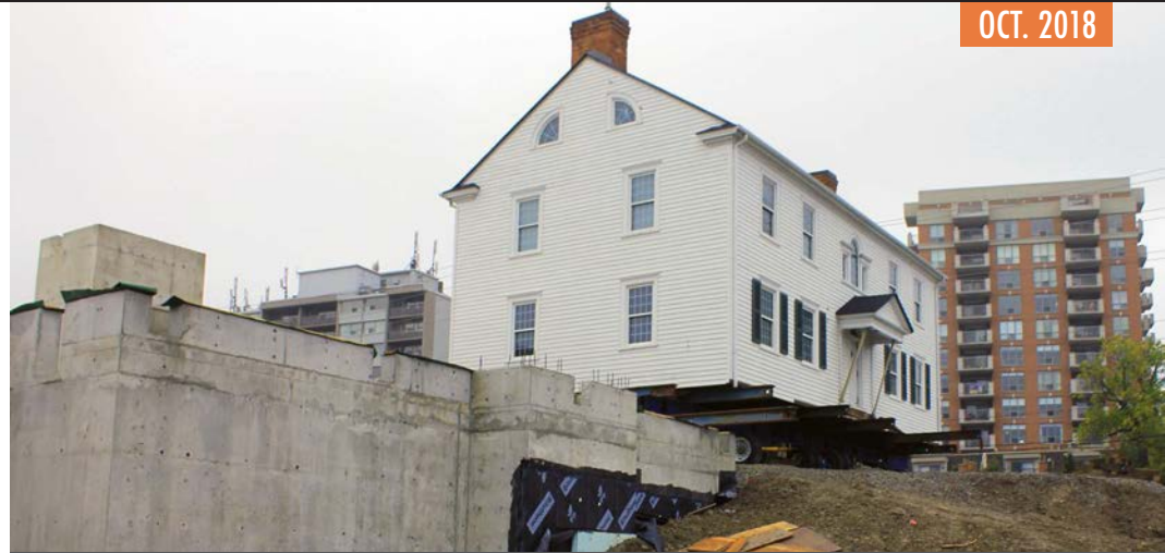
The Brant House is in position to be moved onto its permanent foundation at left, putting it atop the expanded museum with access at street level.
